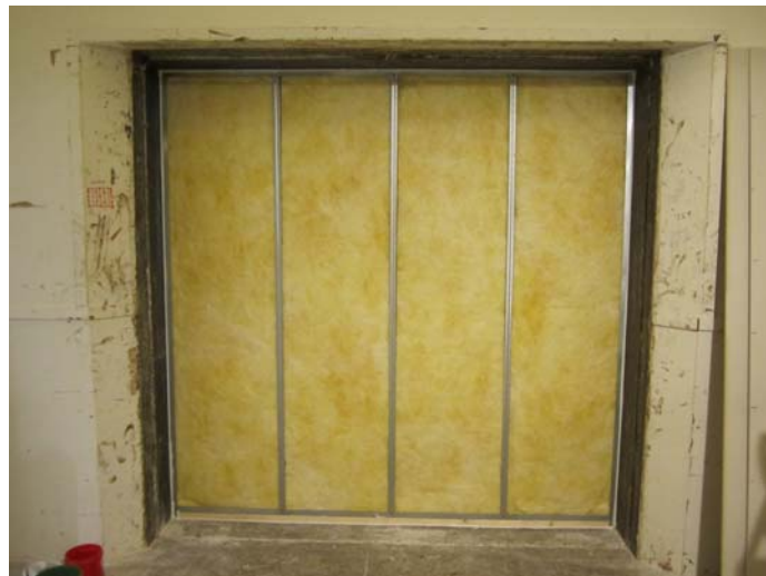
Figure 1: Insulated steel stud frame viewed from source room side
